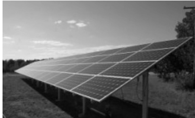
Over 90KW in Solar Installations
