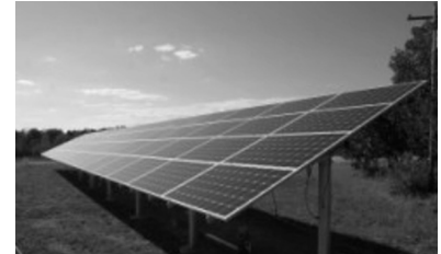
Over 90KW in Solar Installations
